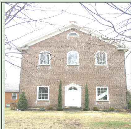
When the windows were replaced for the first time in 1994, the original glass panes were reused. Broken or cracked panes were replaced with the same type of glass used in the original windows, imported from Germany.
